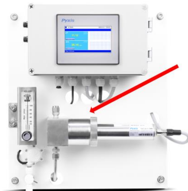
ST-007 Installed with ST-765SS-DCL Downstream of Rotameter
